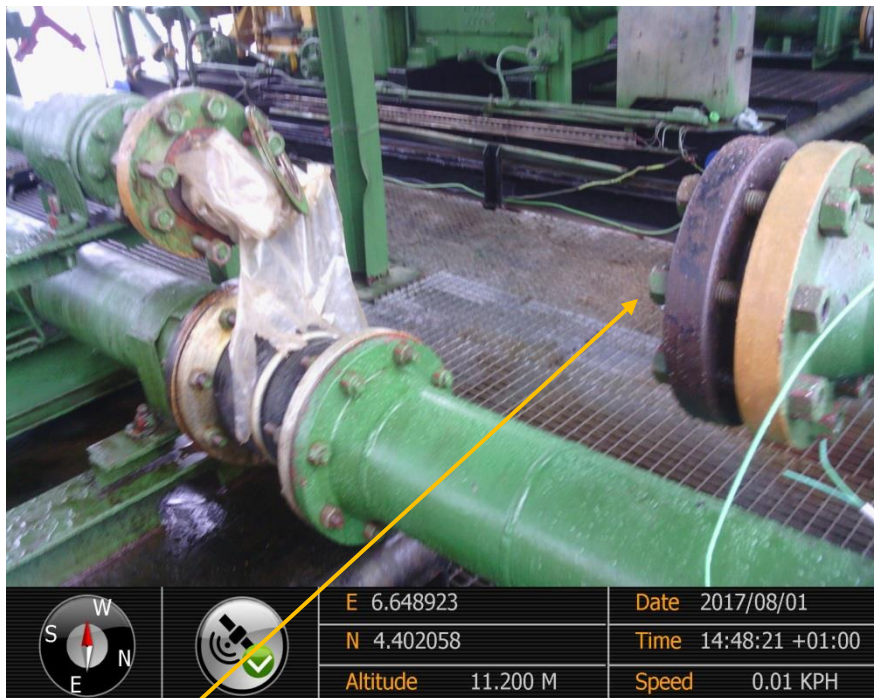
Close-up: Original Position of the Ruptured Flexible Discharge Spool Piece on Belema Flow Station at Belema. Picture was taken during Joint Investigation of 1 st Aug 2017.
