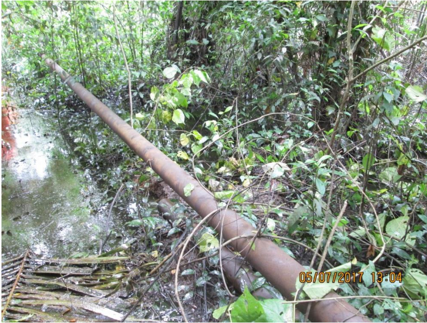
Overview: Part of spill impact on 4" Adibawa Well 2S Flowline Right of Way at Edagberi-Betterland. Picture was taken during Joint Investigation of 5 th July 2017.
