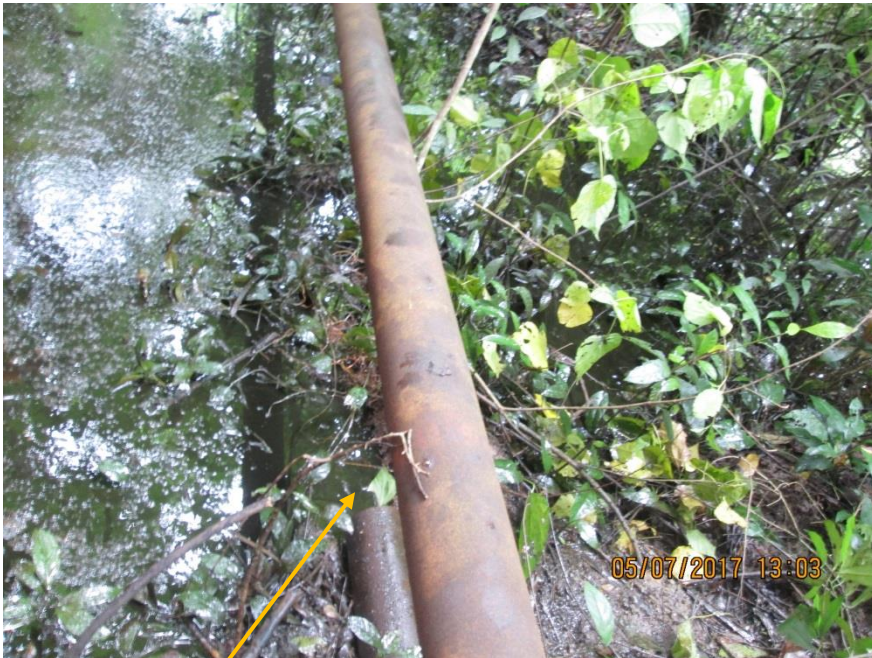
Close-up: Section of Missing Flowline on 4" Adibawa Well 2S Flowline at Edagberi-Betterland. Picture was taken during Joint Investigation of 5 th July 2017.
