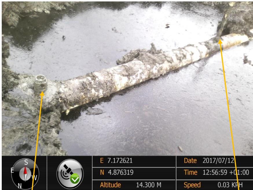
Close-up: Leaking illegal fitting on 12" Imo River-Ogale Pipeline at Komkom. Non-leaking fitting subject to another Joint Investigation Visit.
