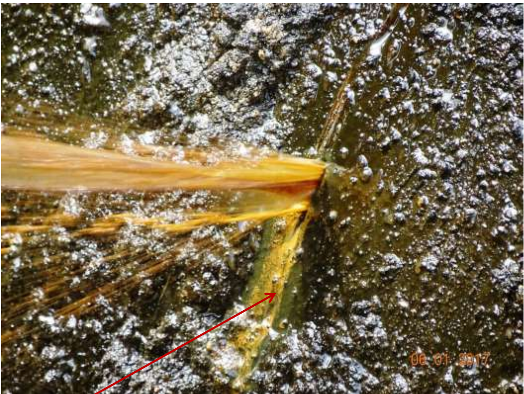
Close-up: Hacksaw cut on 28" Nkpoku-Bomu Trans Niger Pipeline at Kpor. Picture was taken during Joint Investigation of 6 th January 2017.
