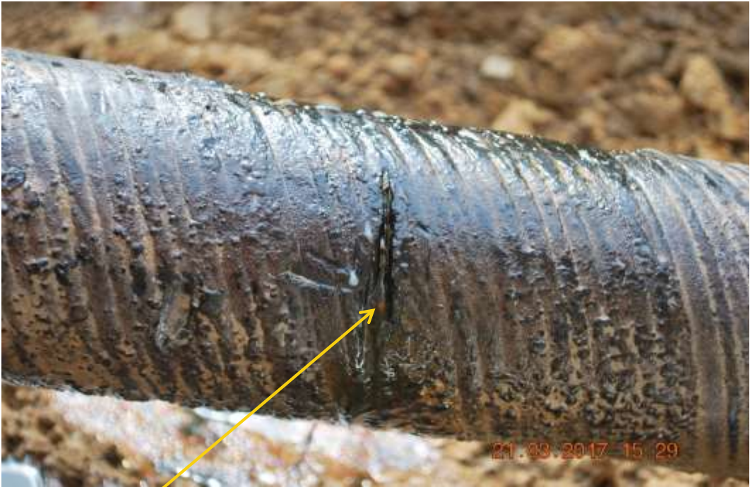
Close-up: 2 nd of 5 Hacksaw cuts on 4" Obele-Ibaa Pipeline at Ibaa. Picture was taken during Joint Investigation of 21 st March 2017.
