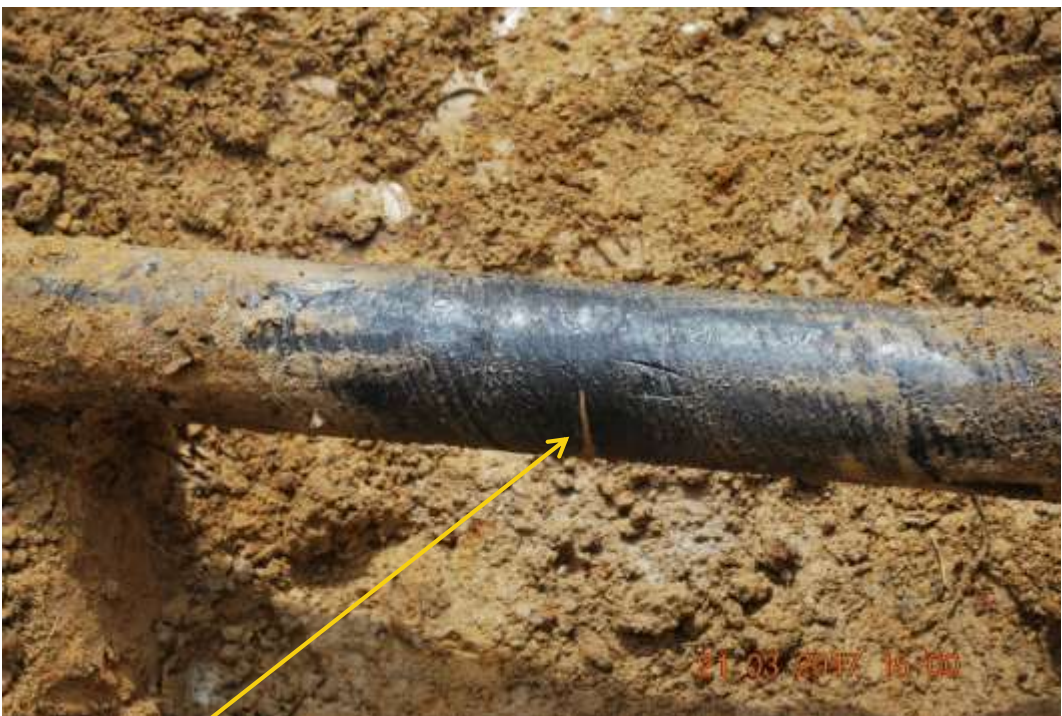
Close-up: 1 st of 5 Hacksaw cuts on 4" Obele-Ibaa Pipeline at Ibaa. Picture was taken during Joint Investigation of 21 st March 2017.
