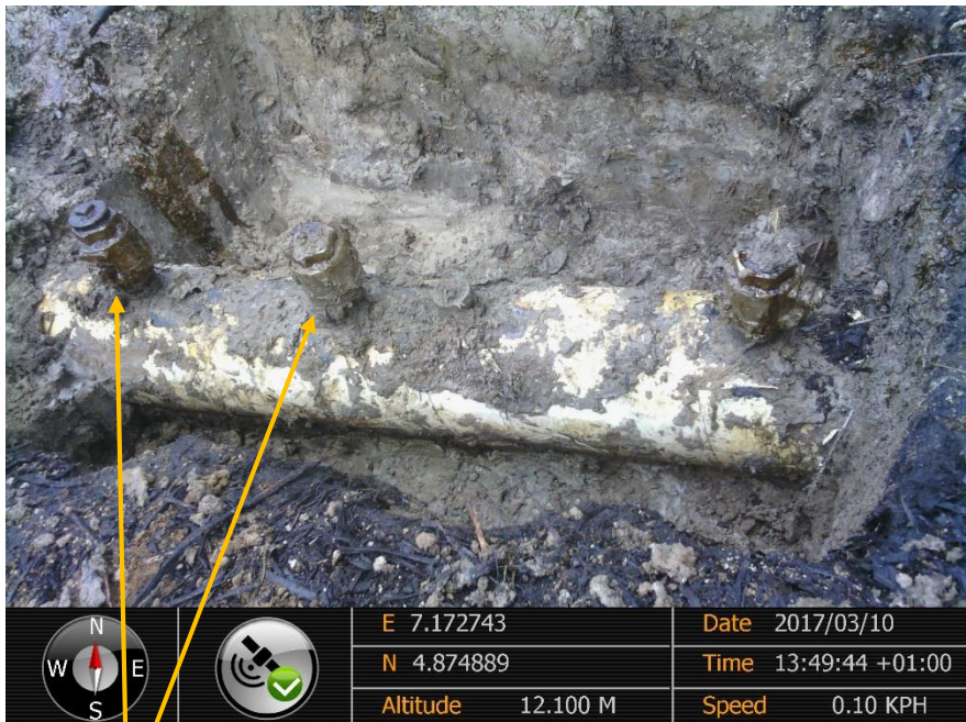
Close-up: Leaking Illegal fittings on 12" Imo River-Ogale Pipeline at Komkom. Picture was taken during Joint Investigation of 10 th March 2017
