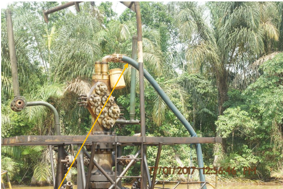
Close-up: 4" illegally attached bunkering hose on Agbaya Well 1 Wellhead at Ogbotobo. Picture was taken during Joint Investigation of 17 th January 2017.
