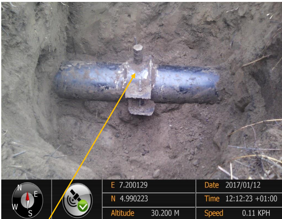
Close-up: Illegal fitting on 6" Imo River Well 59T Flowline at Owaza. Picture was taken during Joint Investigation of 12 th January 2017.
