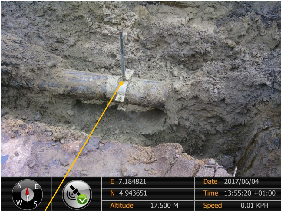
Close-up: Illegal fitting on 12" Imo River-Ogale Pipeline at Umuololo. Picture was taken during Joint Investigation of 4 th June 2017.
