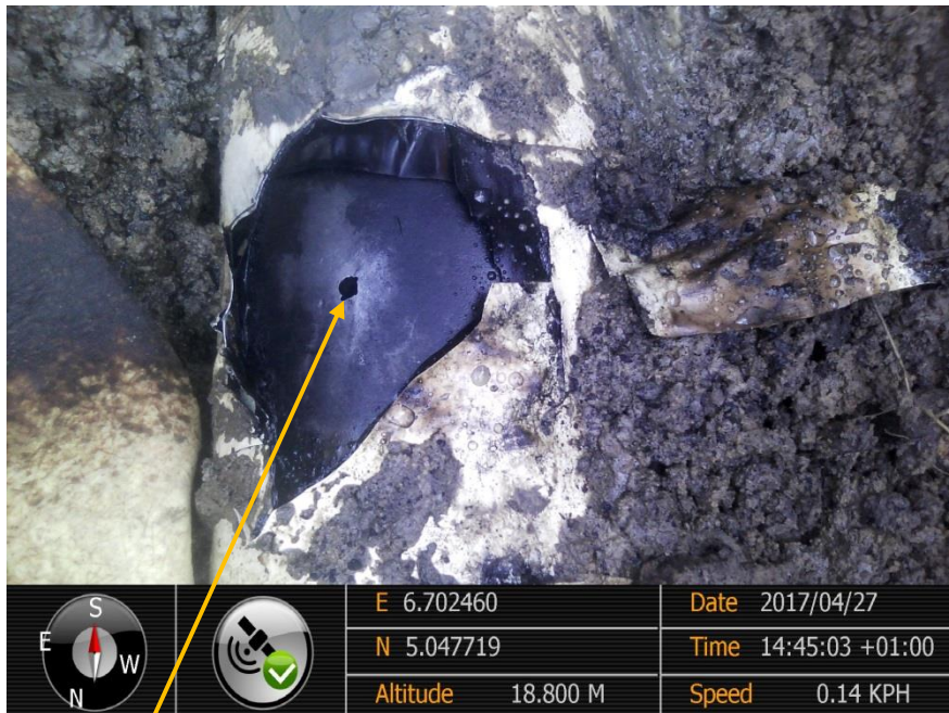
Close-up: Drilled Hole on 8" Mininta-Rumuekpe Bulkline at Ihuaba-Imogu-Elele-Alimini. Picture was taken during Joint Investigation of 27 th April 2017.
