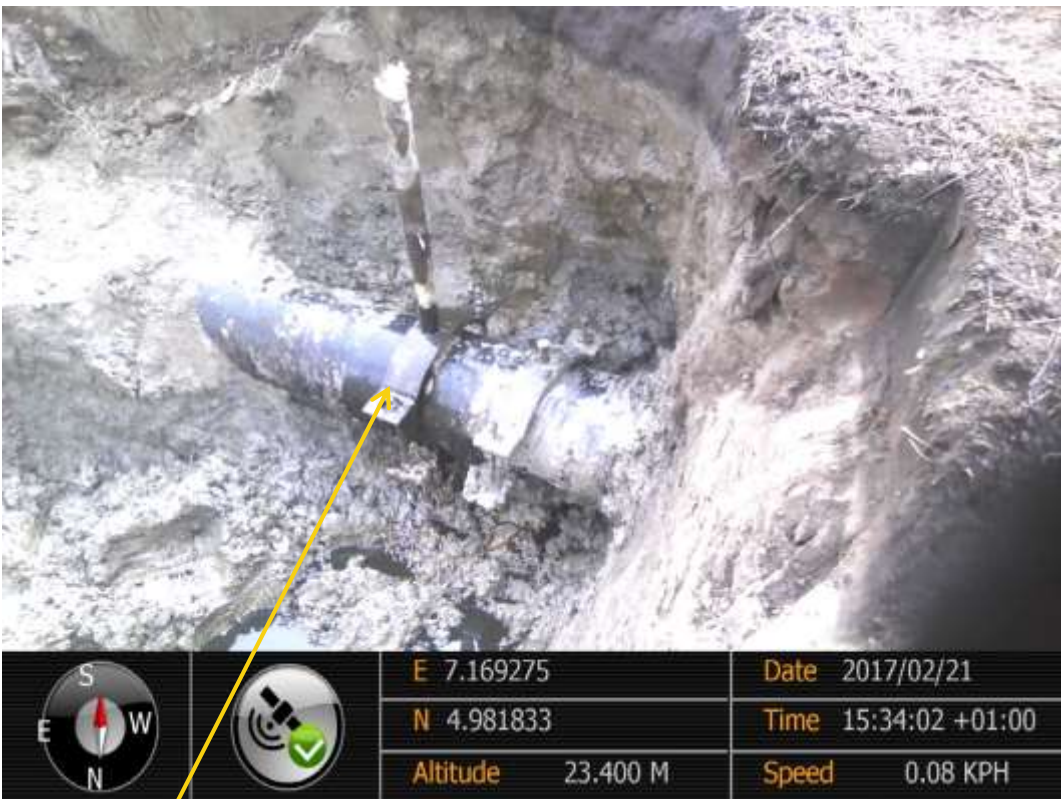
Close-up: Illegal fitting on 12" Imo River2 – Ogale Pipeline at Odagwa. Picture was taken during Joint Investigation of 21 st February 2017.
