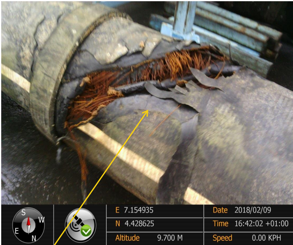
Close-up: Tear on Single Point Mooring one SPM1 at Bonny. Picture was taken during Joint Investigation of 11 th May 2018.
