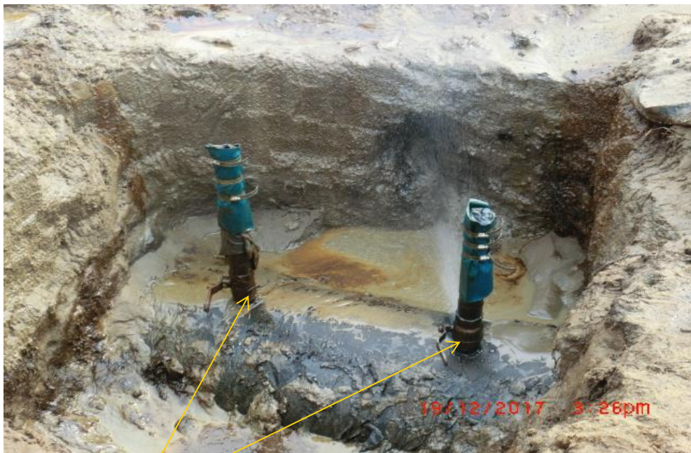
Close-up: Illegal Fittings on 28" Nkpoku- Bomu Pipeline at Eteo. Picture was taken during Joint Investigation of 19 th December 2017.
