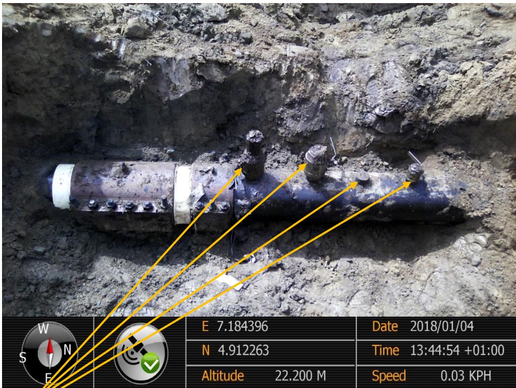
Close-up: Illegal Fittings on 12" Imo River–Ogale Pipeline at Uzuaku. Picture was taken during Joint Investigation of 4 th January 2018.
