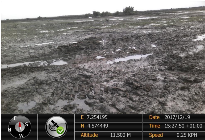
Overview: Part of spill impact on 28" Bomu-Bonny Pipeline Right of Way at Patrick Waterside. Picture was taken during Joint Investigation of 19 th December 2017.
