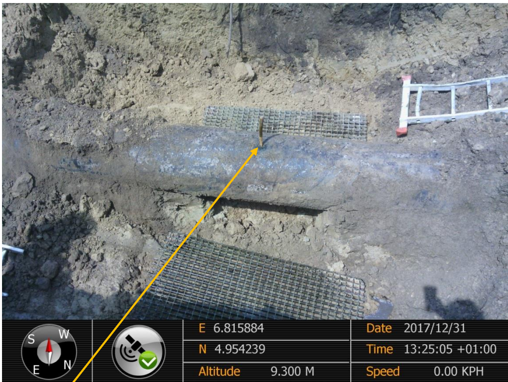
Close-up: Drilled Hole on 20"Rumuekpe-Nkpoku Pipeline at Ibaa. Picture was taken during Joint Investigation of 31 st December 2017.
