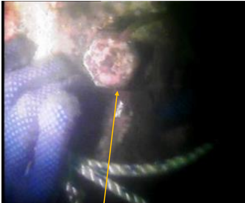
Close-up: Loosed Pressure Release plug on Forcados Terminal Single Point Mooring (SPM)1. Picture was taken during the Initial Site Visit of 28 th December 2017.
