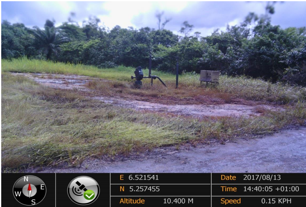
Overview: Part of spill impact on Adibawa North East 1 Well Head at Biseni. Picture was taken during Joint Investigation of 13 th August 2017.
