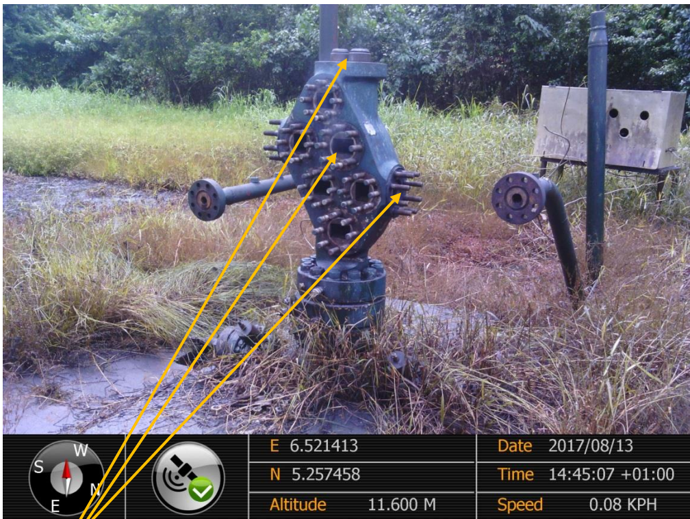
Close-up: Leak Point on Adibawa North East 1 Well Head at Biseni. Picture was taken during Joint Investigation of 13 th August 2017.
