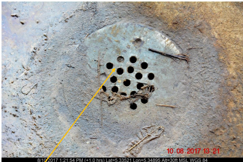
Close-up: Back flow from Continuous Oil Containment Drain Pit on Forcados KTI Emulsion Heater Treatment Unit at Ogulagha. Picture was taken during Joint Investigation of 10 th JAugust 2017.
