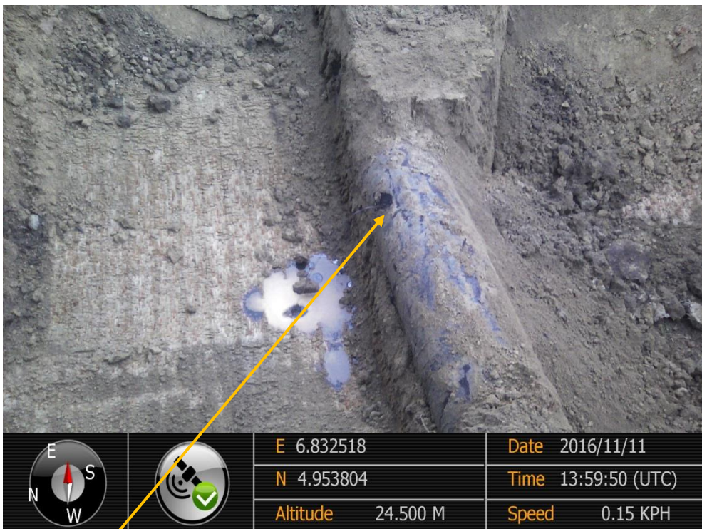
Close-up: Drilled hole on 20" Rumuekpe-Nkpoku Trans Niger Pipeline at Ibaa. Picture was taken during Joint Investigation of 11 th November 2016.
