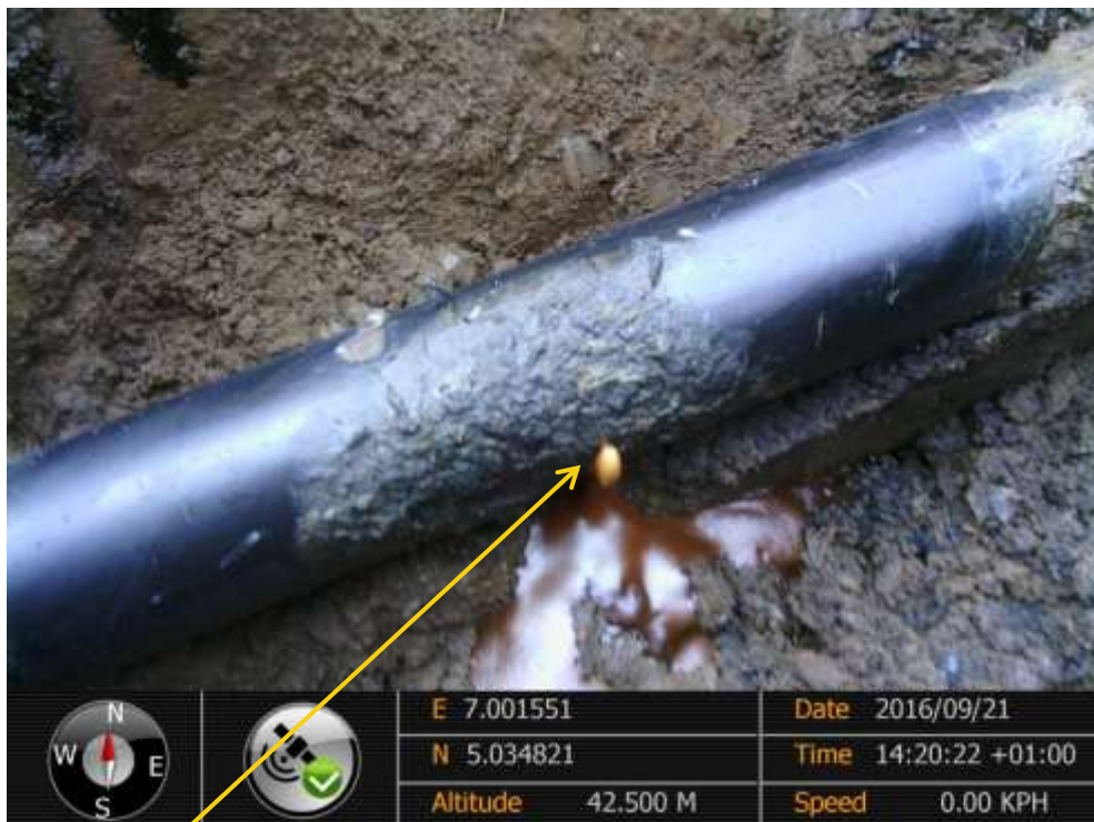
Close-up: Leak point on Otamiri Well5 Flowline at Abara. Picture was taken during Joint Investigation of 21 st September 2016.
