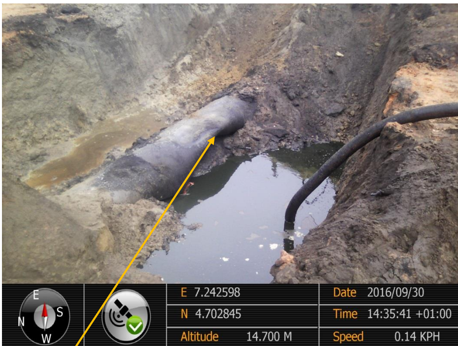
Close-up: Inward dent on 28" Nkpoku-Bomu Pipeline at Gio. Picture was taken during Joint Investigation of 30 th September 2016.
