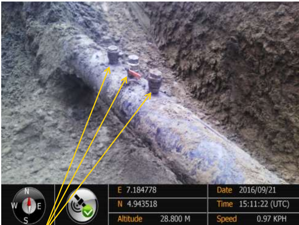
Close-up: Illegal fittings on 12" Imo River – Ogale Pipeline at Owaza. Picture was taken during Joint Investigation of 21 st September 2016.
