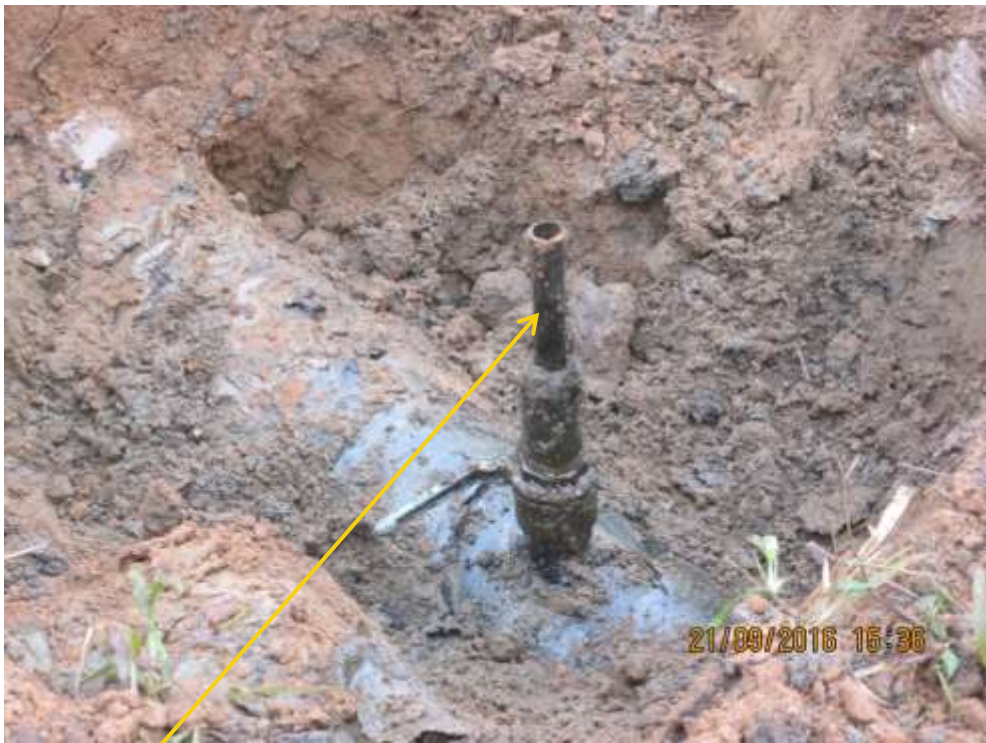
Close-up: Illegal fitting on 12" Imo River – Ogale Pipeline at Ogale. Picture was taken during Joint Investigation of 21 st September 2016.
