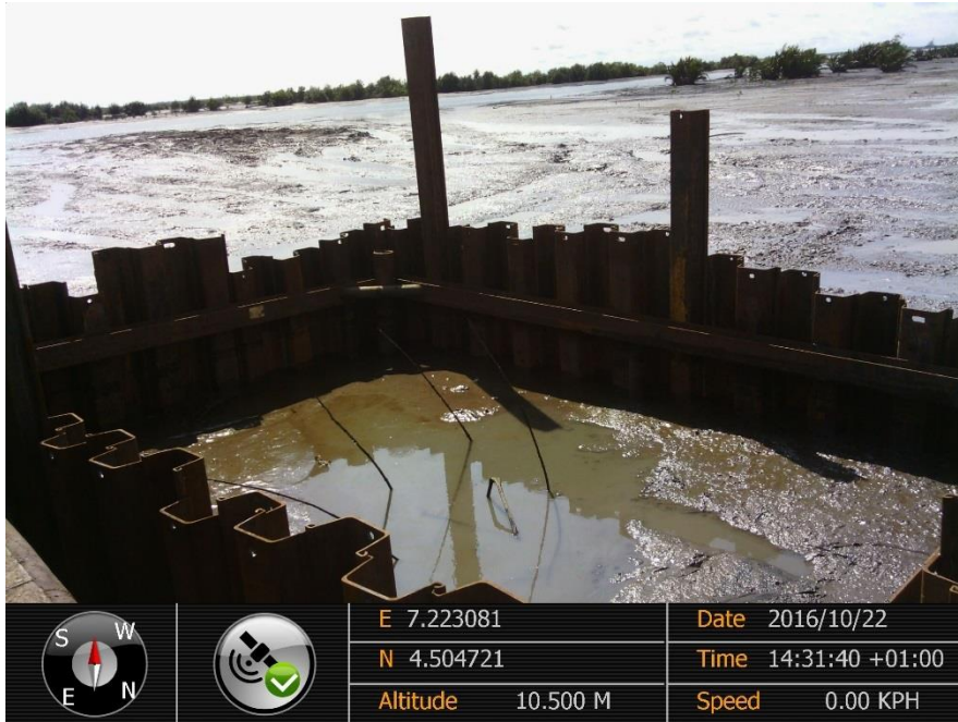
Overview: Part of spill impact 28" Bomu-Bonny Pipeline at Okolo Launch. Picture was taken during Joint Investigation of 22 nd October 2016.
