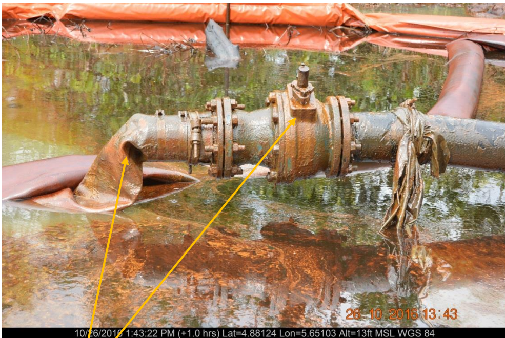
Close-up: Illegally attached flexible hose and 6" valve on 6" Kanbo Well 7S Flowline at Agbidiama. Picture was taken during Joint Investigation of 26 th October 2016.
