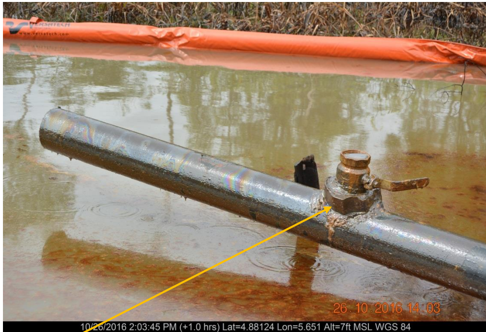
Close-up: Illegally attached 3" valve on 6" Kanbo Well 9T Flowline at Agbidiama. Picture was taken during Joint Investigation of 26 th October 2016.
