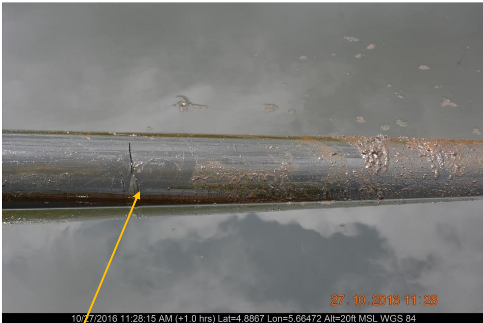
Close-up: Hacksaw cut on 6" Kanbo Well 6T Flowline at Agbidiama. Picture was taken during Joint Investigation of 27 th October 2016.
