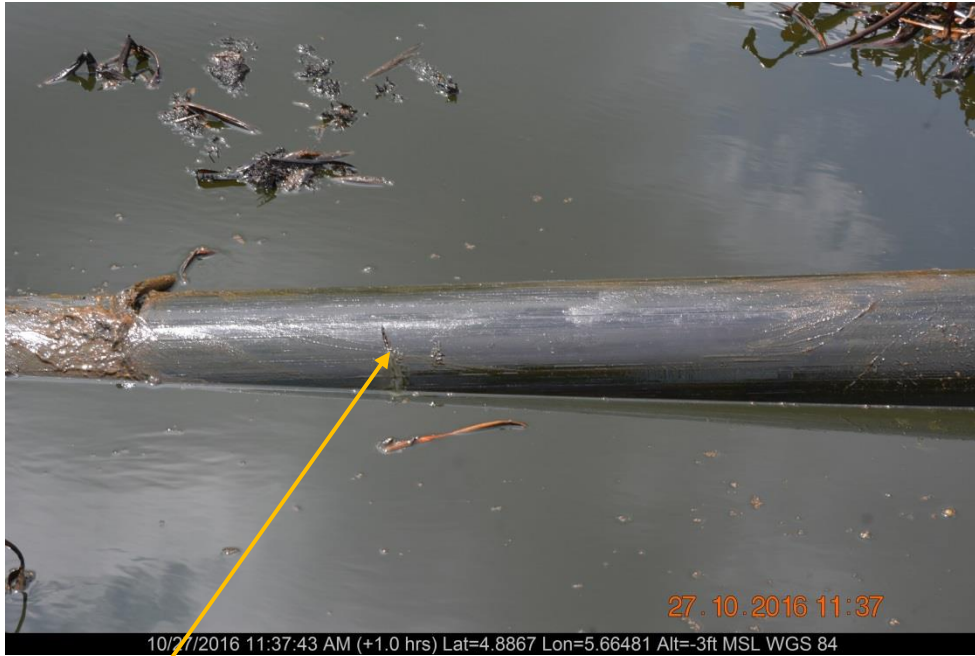
Overview: Hacksaw cut on 6" Kanbo Well 6T Flowline at Agbidiana. Picture was taken during Joint Investigation of 27 th October 2016.
