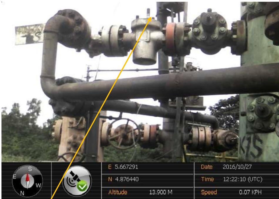
Close-up: Position of stolen CCU actuator on Kanbo Wells - 7L/S and 9T Wellheads Cluster at Agbidiana. Picture was taken during Joint Investigation of 27 th October 2016.
