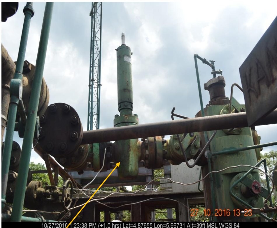
Close-up: Tampered CCU actuator on Kanbo Wells - 7L/S and 9T Wellheads Cluster at Agbidiana. Picture was taken during Joint Investigation of 27 th October 2016.
