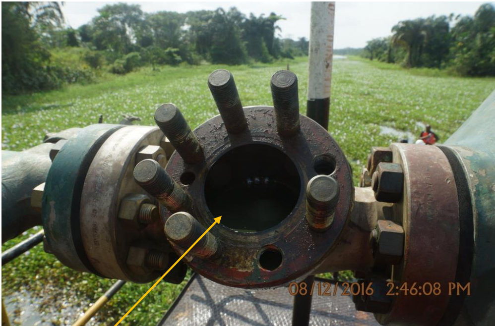
Close-up: Position of stolen surface safety valve (AVA) on Benisede Well 6S Wellhead at Ojobo. Picture was taken during Joint Investigation of 8 th December 2016.
