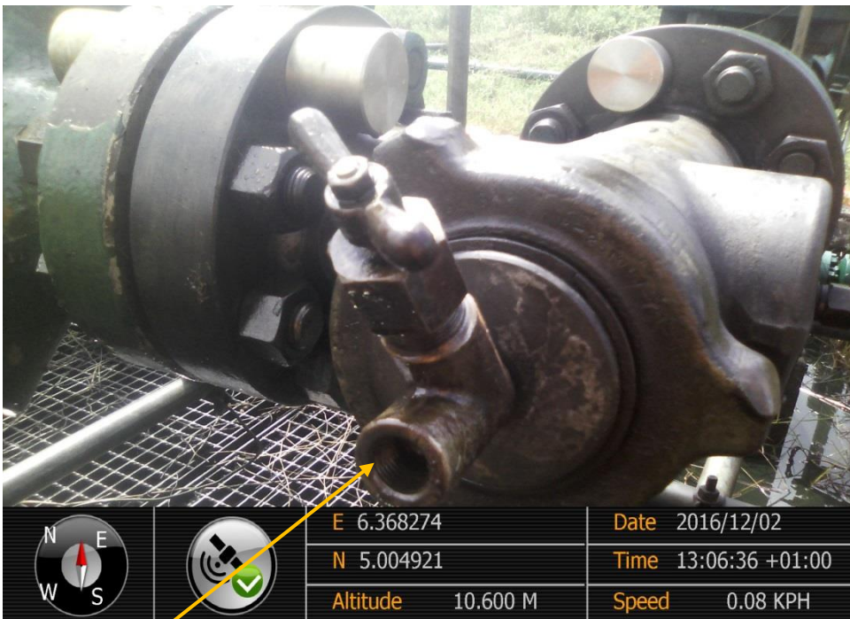
Close-up: Tampered Cork valve on Etelebou Well-11T Well head at Akenfa. Picture was taken during Joint Investigation of 2 nd December 2016.
