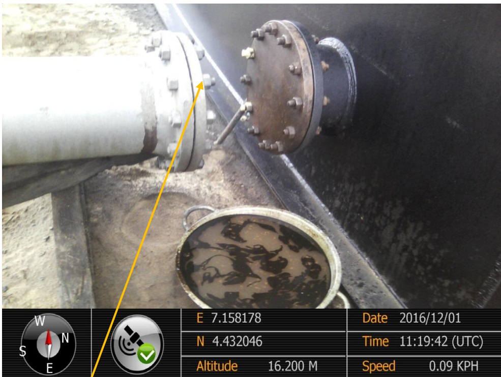
Close-up: Leaking flange on Bonny Terminal tank15-10'' drainline flange at Bonny. Picture was taken during Joint Investigation of 1 st December 2016.
