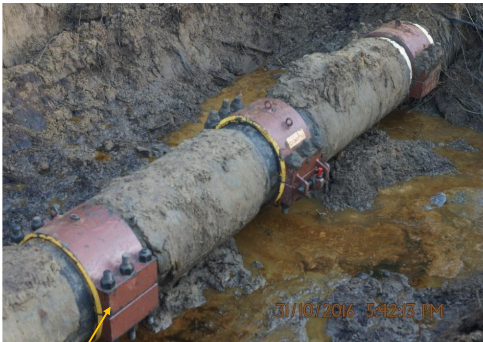
Close-up: Tampered Clamp on 20" Otumara-Escravos Pipeline at Ogidigben. Picture was taken during Joint Investigation of 31 st October 2016.
