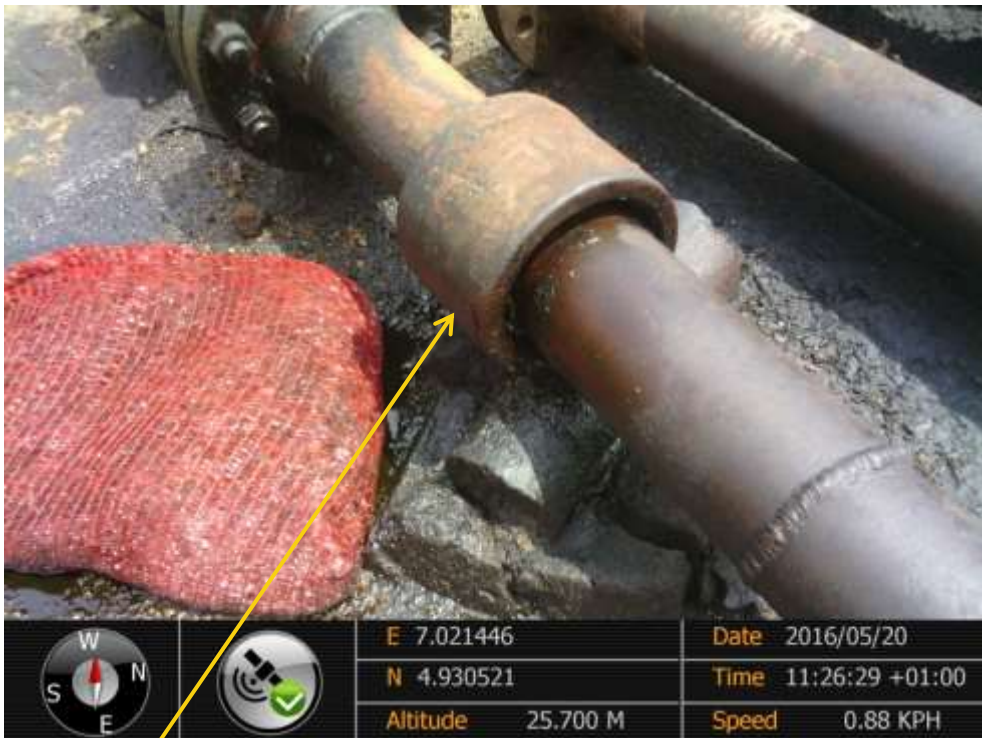
Close-up: Cathodic Leak joint damaged by fire on Agbada2 Well 41/42/43 Cluster at Omuohia/Omuokoji. Picture was taken during Joint Investigation of 20 th May 2016.
