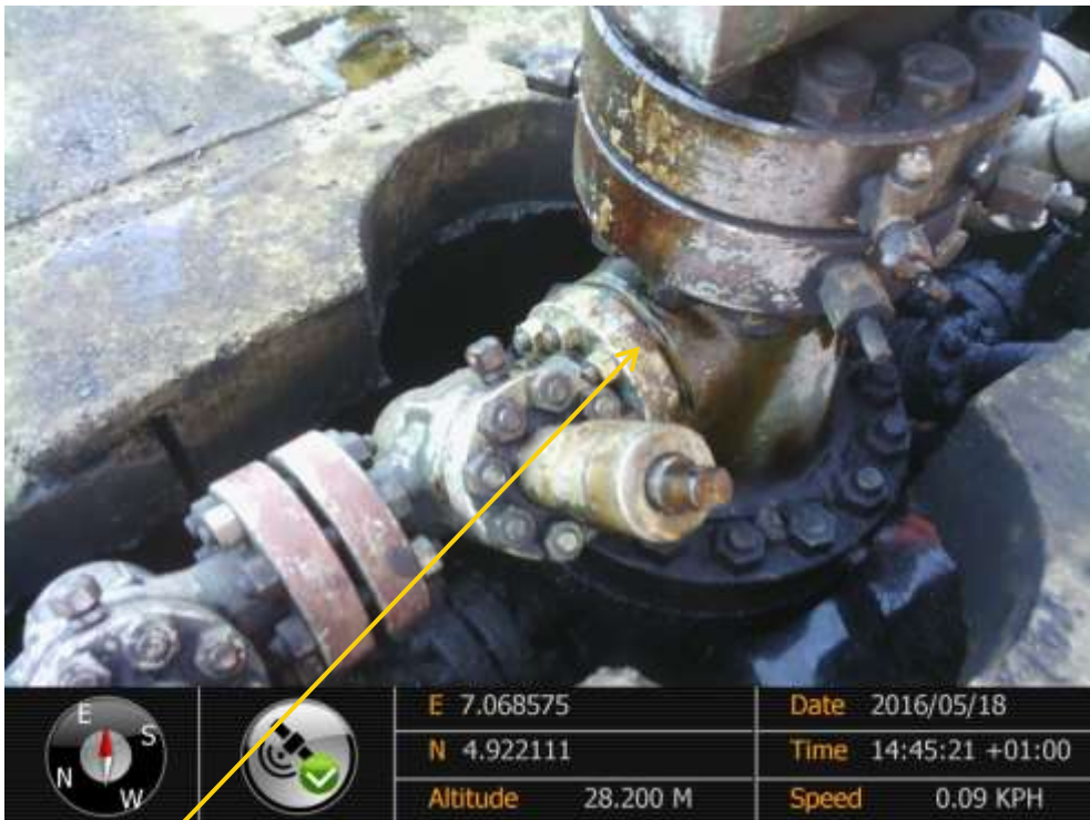
Close-up: Leak on Obigbo Well28 at Imeh. Picture was taken during Joint Investigation of 18 th May 2016.
