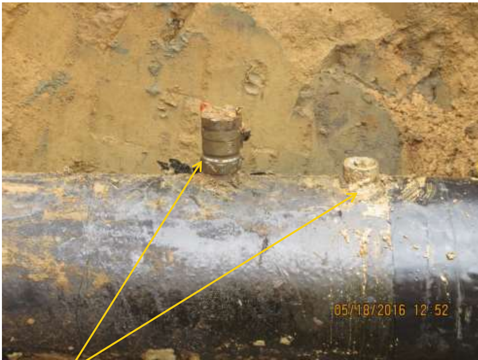
Close-up: Illegal fittings on 12" Imo River – Ogale Pipeline at Owaza. Picture was taken during Repair Operation on 18 th May 2016.
