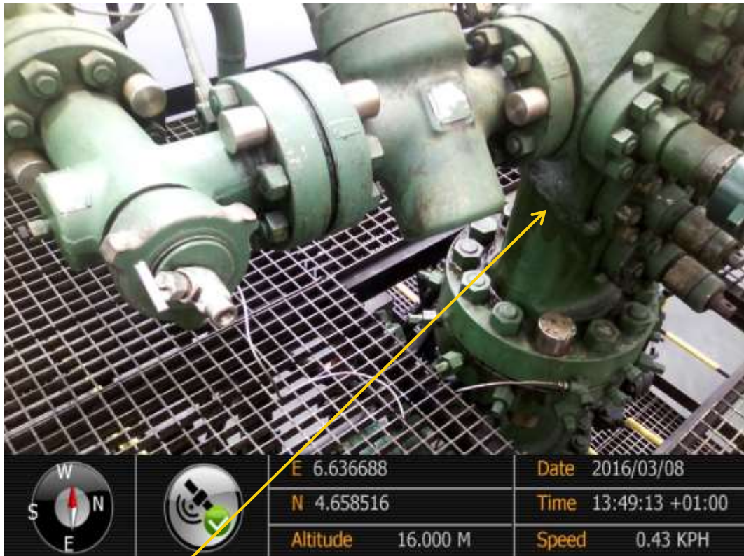
Close-up: Oil stains observed on Soku Well 21L Wellhead at Soku. Picture was taken during Joint Investigation of 8 th March 2016.
