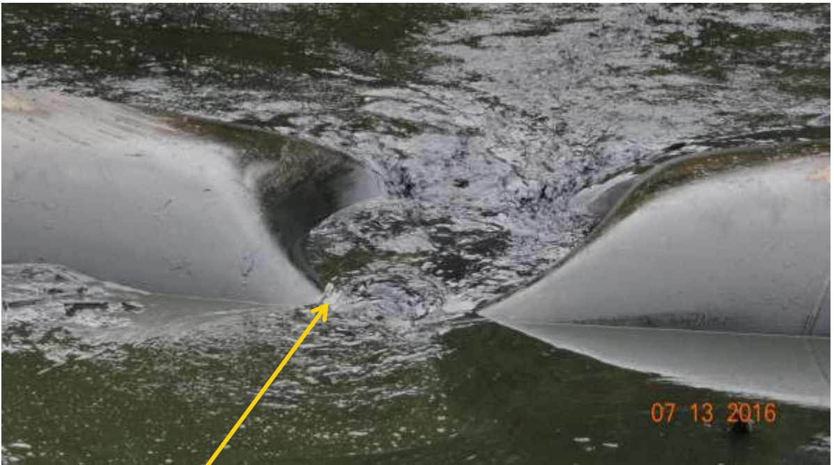
Close-up: Spill point on 48" Forcados Export Pipeline at Ogulagha. Picture was taken during Pipeline Repair works on 13 th July 2016.
