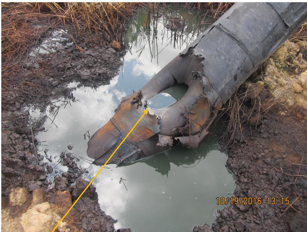
Close-up: Inward dent, explosive tear on 20" Kolocreek-Rumuekpe Pipeline Riser at Aminigboko. Picture was taken during Joint Investigation of 19 th October 2016.
