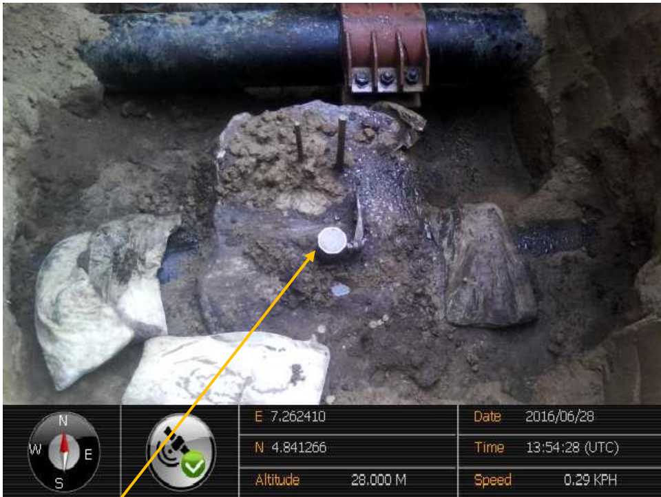
Close-up: Illegal fitting on 8" Afam Well 27 T Flowline at Ayama. Picture was taken during Joint Investigation of 28 th June 2016.
