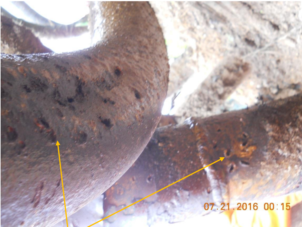
Close-up: Irregular holes and Marks on Obigbo North Well 26T_18S Flowlines at Umuwalia. Picture was taken during Joint Investigation of 21st July 2016.
