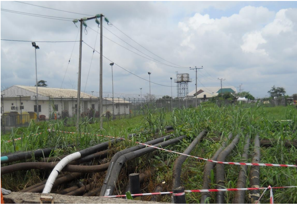
Overview: Part of spill impact on Obigbo North Well 26T_18S_20T_three disused Flowlines at Umuwalia. Picture was taken during Joint Investigation of 21st July 2016.
