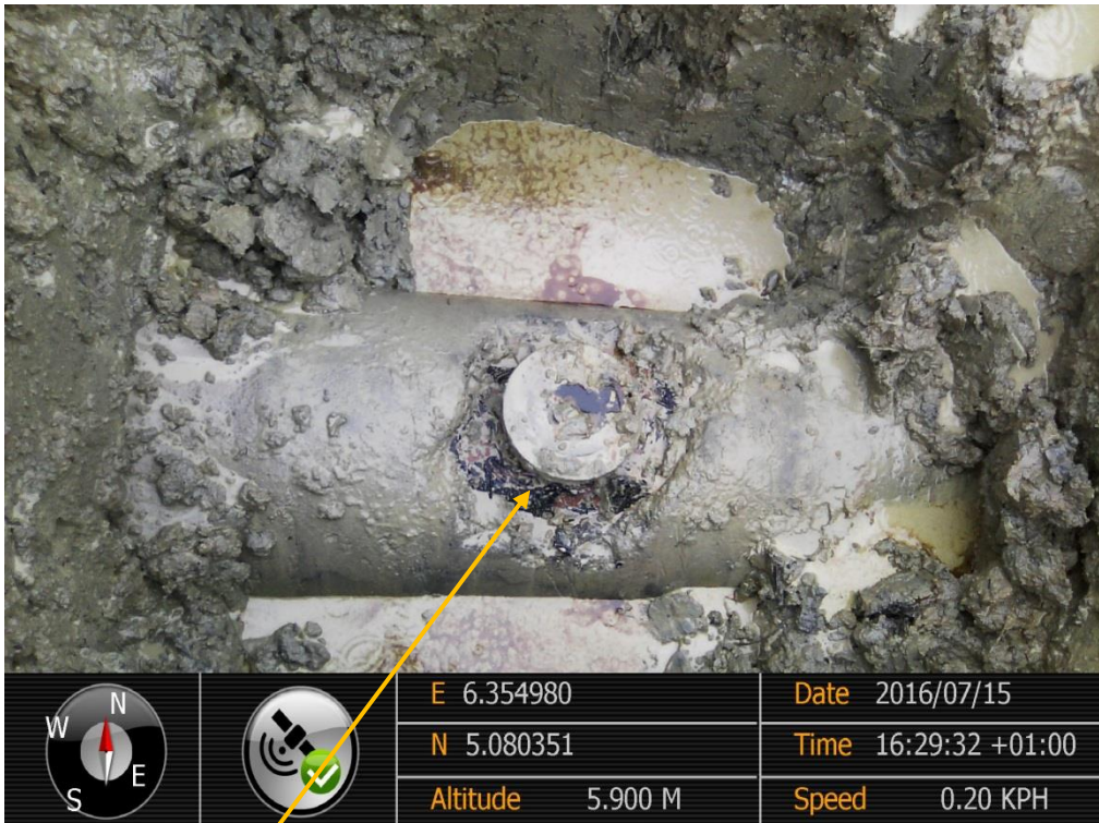
Close-up: Illegal fitting on 16" Zarama-Gbaran CPF Bulkline at Okotiana. Picture was taken during Joint Investigation of 15 th July 2016.
