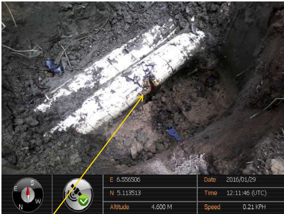
Close-up: Hacksaw cut (Point 1) on Ubie Well5LS Flowline at Idu Ekpeye. Picture was taken during Joint Investigation of 29 th January 2016.
