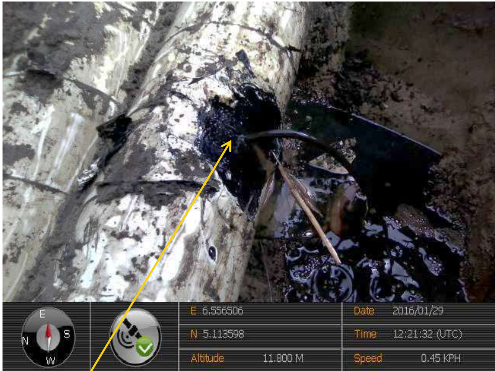
Close-up: Hacksaw cut (Point 2) on Ubie Well5LS Flowline at Idu Ekpeye. Picture was taken during Joint Investigation of 29 th January 2016.
