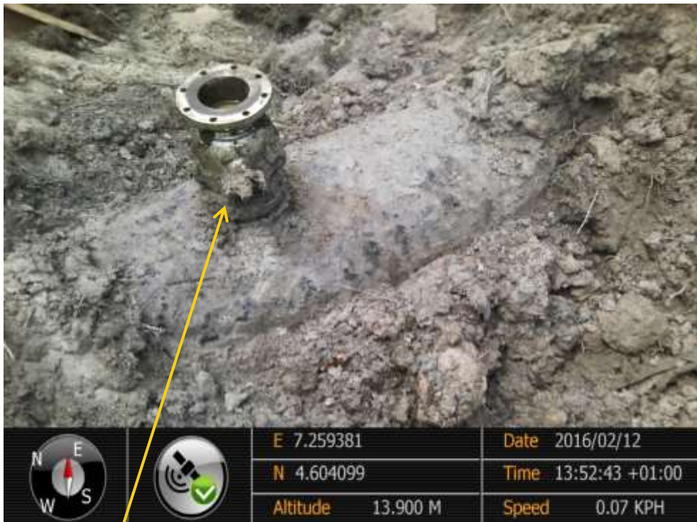
Close-up: Illegal fitting on 28" Bomu-Bonny Pipeline at Bodo City. Picture was taken during Joint Investigation of 12 th February 2016.
