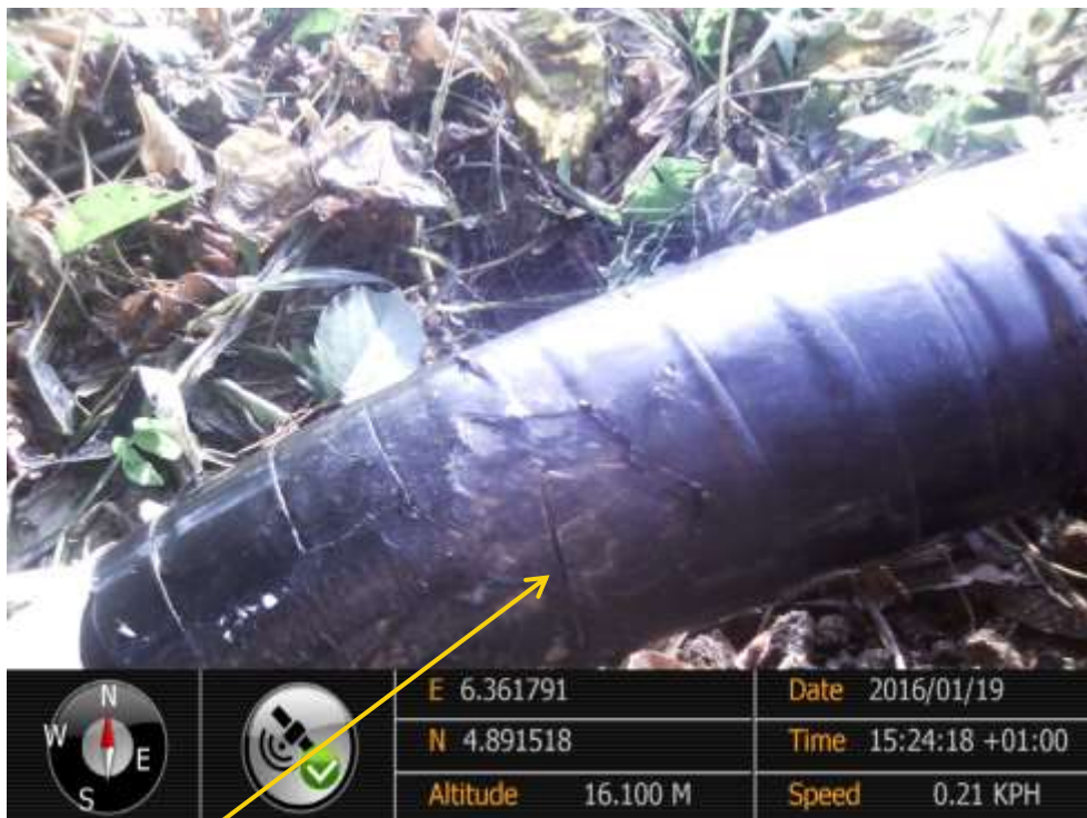
Close-up: Hacksaw cut on KoloCreek Well3T Flowline at Otusega. Picture was taken during Joint Investigation of 19 th January 2016.
