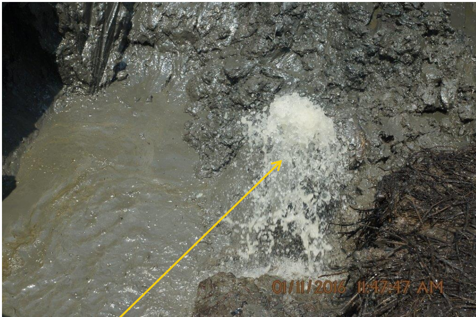
Close-up: Oily Water bubbling out from Illegal Fitting on 20" Otumara-Escravos Pipeline at Ugboegungun. Picture was taken during Joint Investigation of 1 st November 2016.
