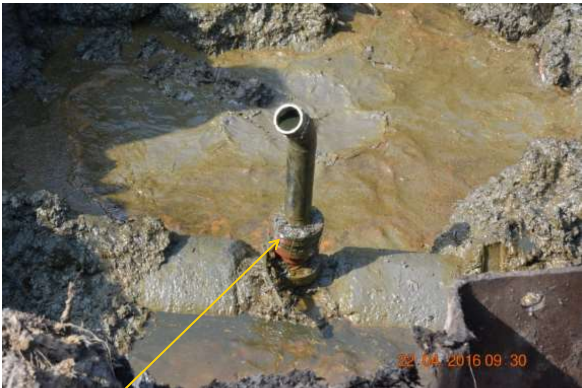
Close-up: Illegal fitting on 20" Opukushi – Brass Creek Pipeline at Tamogbene. Picture was taken during Joint Investigation of 20 th April 2016.
