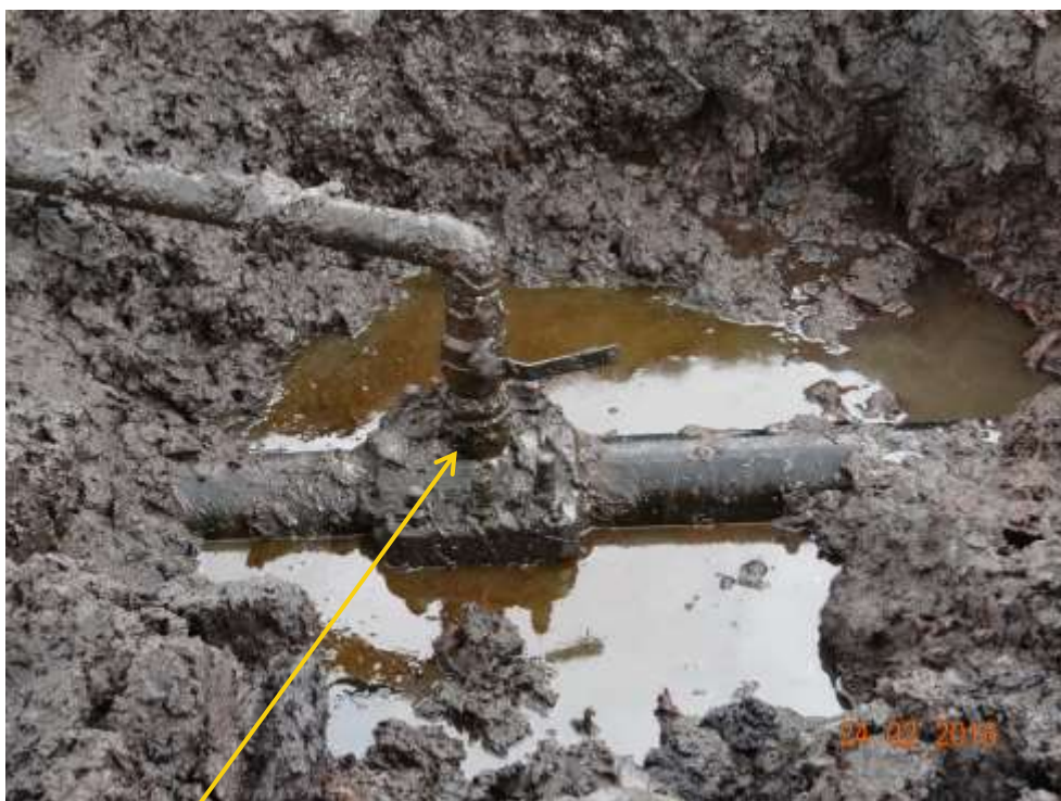
Close-up: Illegal fitting on Belema Well1L 4" Flowline at Belema. Picture was taken during Joint Investigation of 24 th February 2016.
