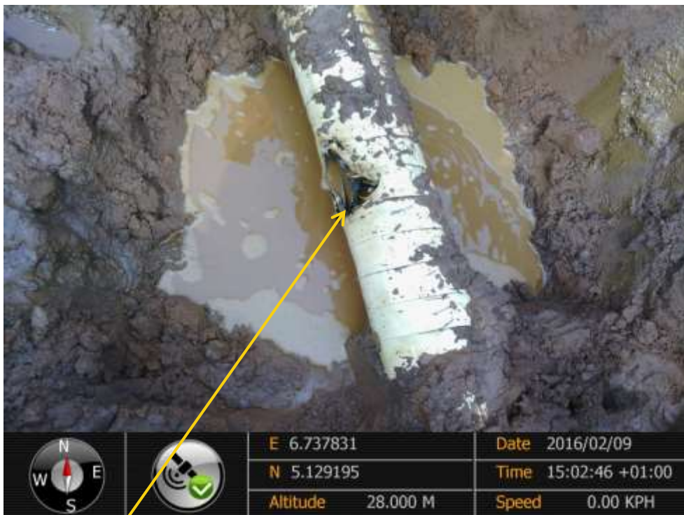
Close-up: Damage due to 3 rd party impact on 6" Mini Nta – Ahia Bulkline at Akpabu. Picture was taken during Joint Investigation of 9 th February 2016.
