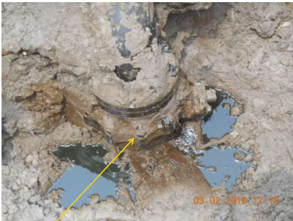
Close-up: Illegal fitting on 28" Nkpoku - Bomu Pipeline at Kporghor/Gbam. Picture was taken during Joint Investigation of 3 rd February 2016.
