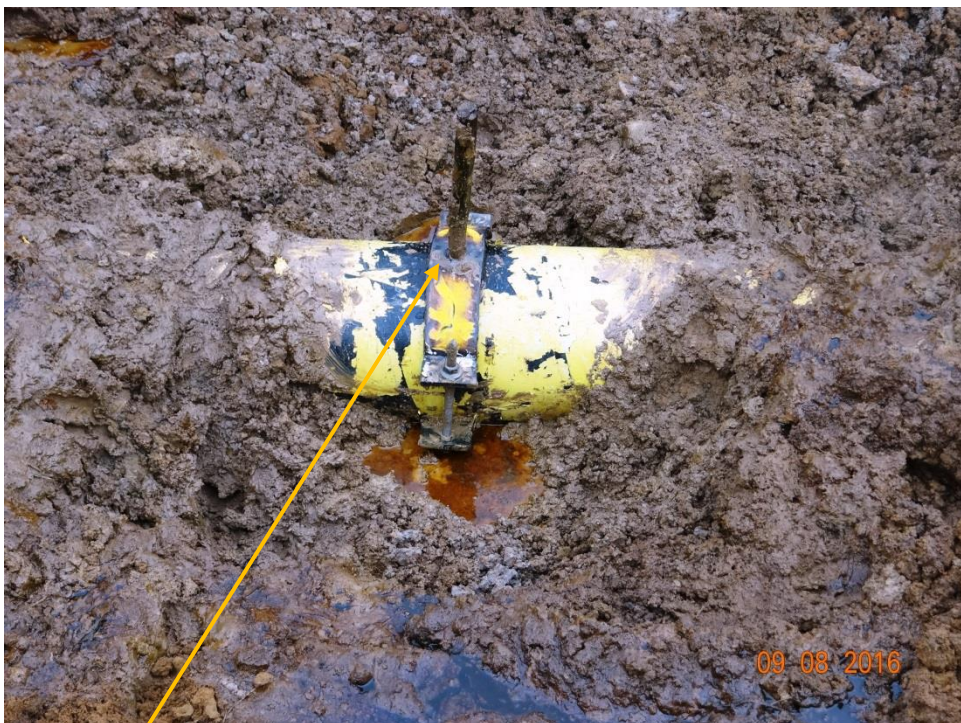
Close-up: Illegal fitting on 12" Imo River 2-Ogale Trans Niger Pipeline at Owaza. Picture was taken during Joint Investigation of 9 th August 2016.
